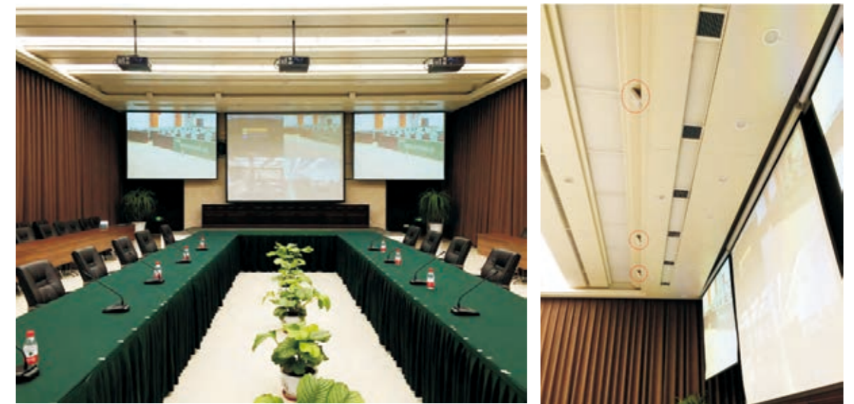
WDC-900 | Power Supplier of Shouguang City, Shandong Weifang
